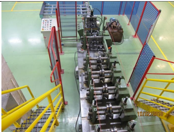
Hydraulic cutting unit after the roll forming machine (Stam)
